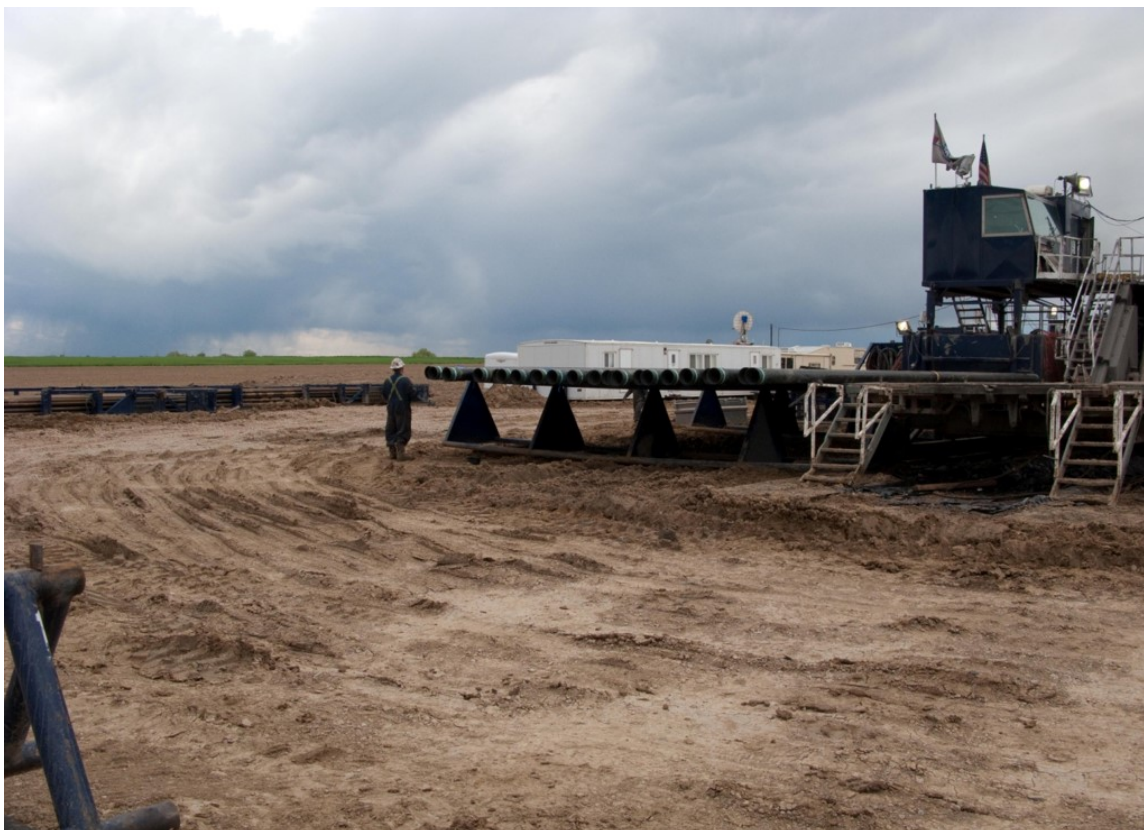
Figure 2-7. Sections of surface casing lined up and being prepared for installation at a well site in Colorado.
